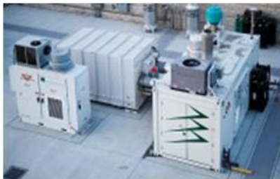
300 kW power plant at a wastewater plant
