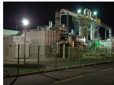
4.8 MW utility owned power plant
