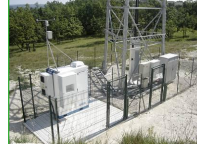
France – Bouygues Telecom
