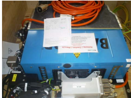
August 03rd 2007 Arrival of the Nucellsys systems and the batteries from MS-DEA
