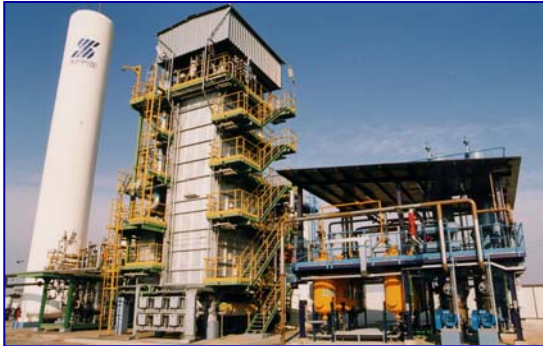
On site H2 production
