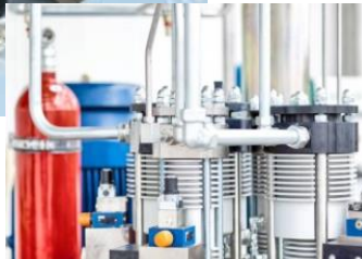
Linde: Ionic H2-Compressor
