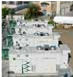
Sierra Nevada Brewery Nat Gas and BioGas CHP
