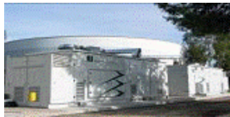
Santa Barbara WWT Plant BioGas CHP
