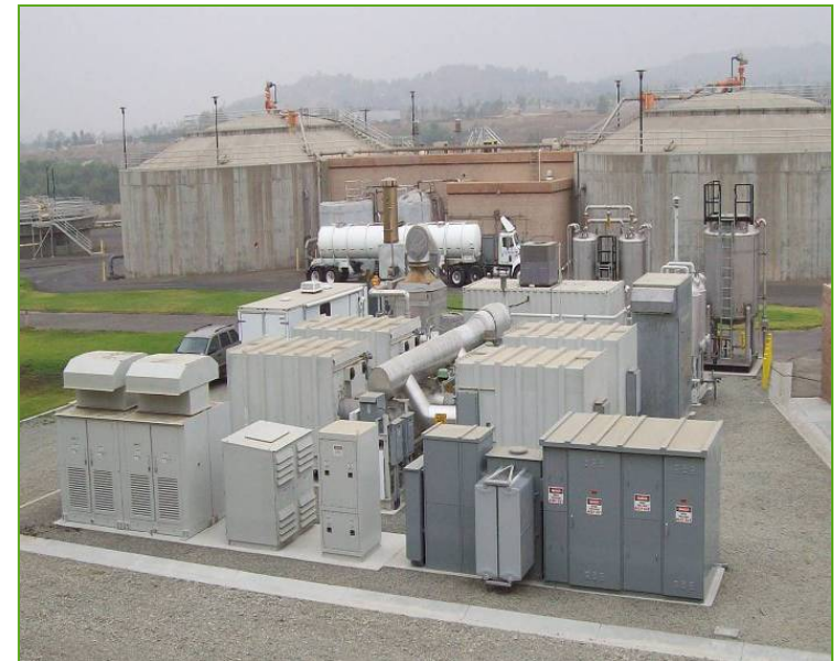
1 MW DFC1500 at a wastewater treatment facility in southern CA
