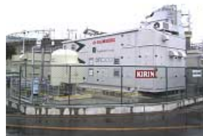
Kirin Brewery BioGas and Propane CHP
