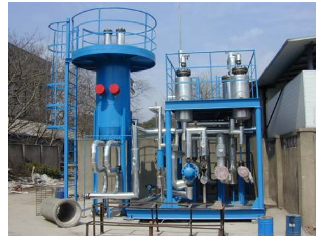
The hydrogen source system of natural gas reforming- Jiaotong university
