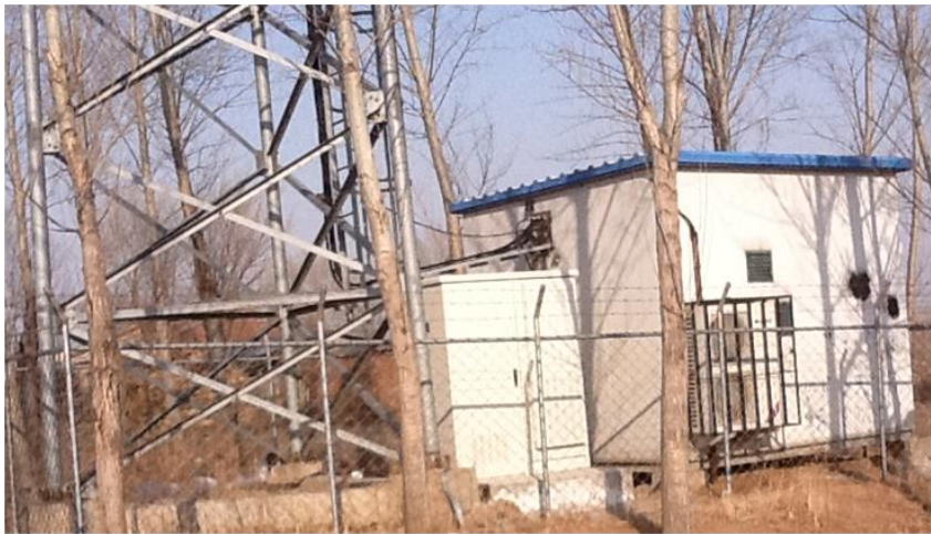
VN Tech backup power system
